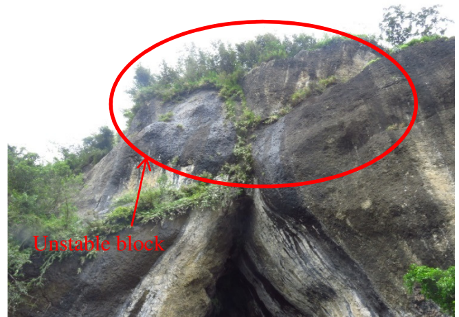
Figure 11. Unstable block at Baxian Cave
